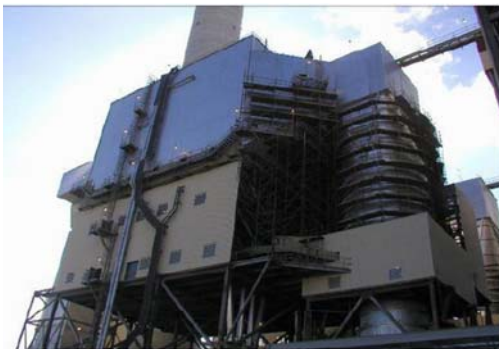
Fig. 2 Desulphurization and Dedust Island of Puerto Rico Power GUAYAMA Plant in the USA
