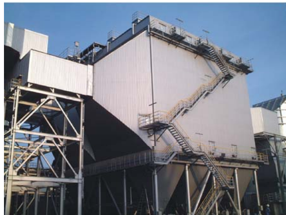
Fig. 7 View of the #6 low-low temperature ESP at Tosoh Nanyo
