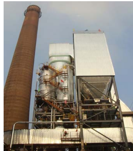
Fig. 2 SanGang 180 m 2 Dry FGD System
