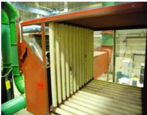
Fig. 7 Filter top with pulse pipes and outlet dampers
