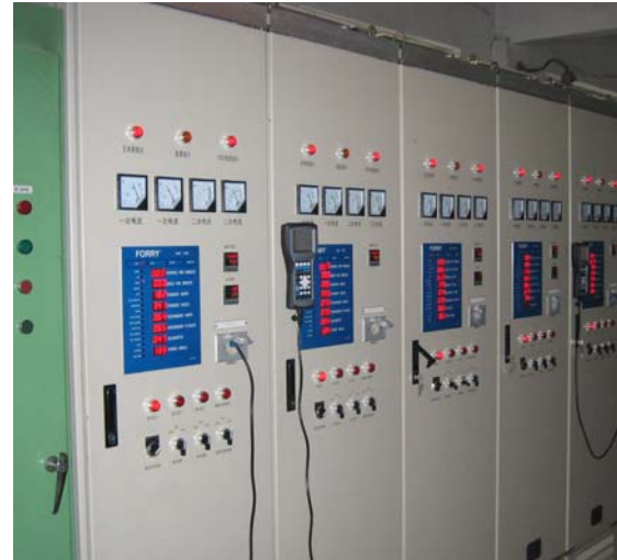
Fig. 3 New AVC XM Cabinets with optional Flush Mounted Displays. Note the analog meters are still best practice for certain troubleshooting techniques.
