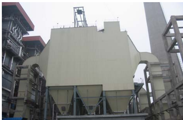
Fig. 3 Changzhou Guangyuan Cogeneration Co., Ltd. Moving Electrode Type ESP for CFB No. 5 Boiler
