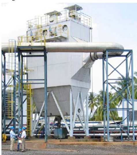
Fig. 7 ESP Installation in Guatemala
