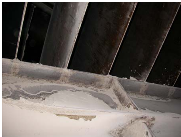
Fig.3 Fouling on the support structure
