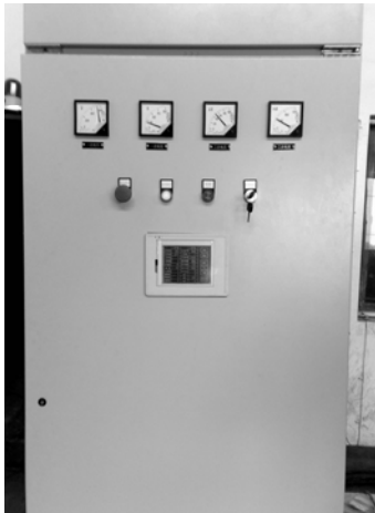
Fig. 8 The door graph of control cabinet
