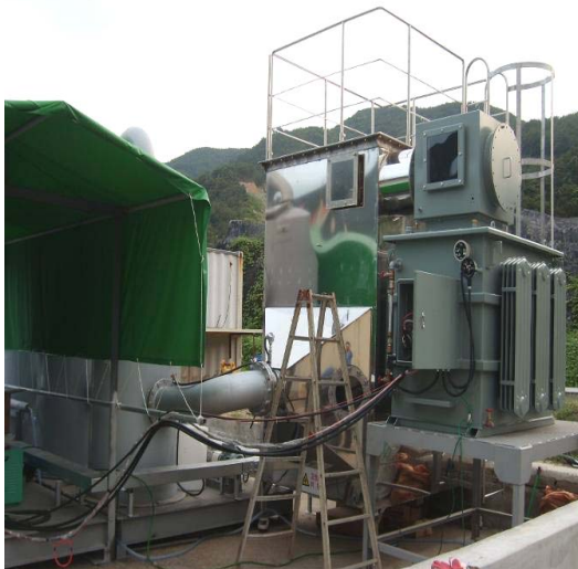
Fig. 3: Pilot system was installed for flue gas odor treatment test at waste food dry recycling plant
