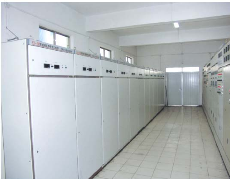
Figure 38, F-Series Power Supply (12 Units on Left Side) and Power Frequency Power
