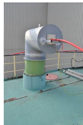
Fig. 4: Example of an HV connection
