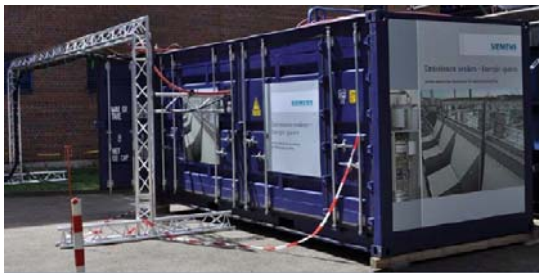
Fig. 1: Mobile test system installation
