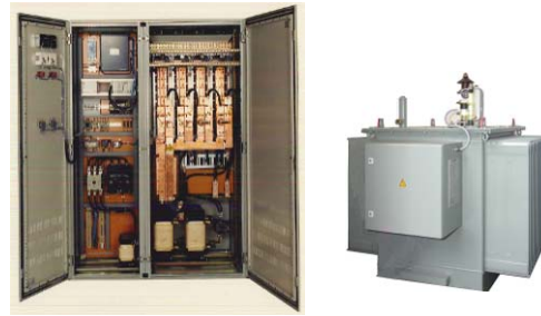
Fig. 3-1: VARIOVOLT control cubicle and HV transformer rectifier (1989)
