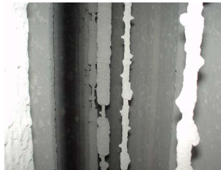
Fig. 7-2: Figure not cleaned discharge electrode
