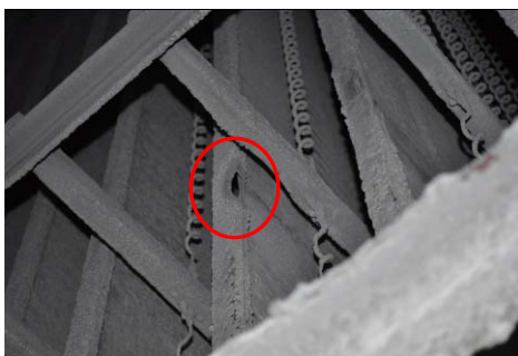
Fig. 7-1: Discharge frame misalignment with local flash-over marks
