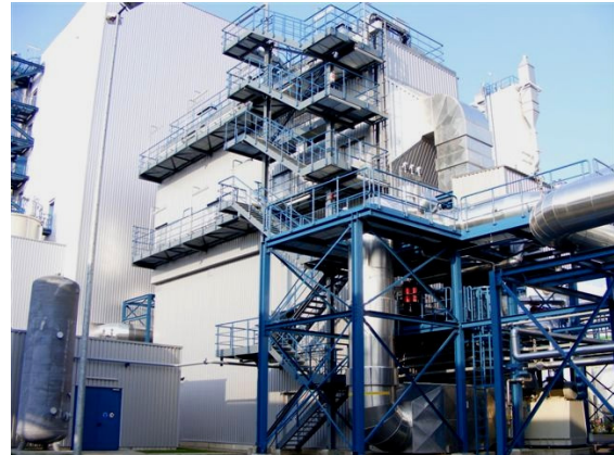
Fig. 2: Photograph of the three-field ESP at Schwarze Pumpe.
