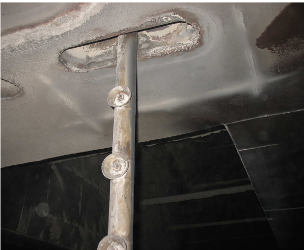
Fig. 2. Injection pipes (lances) inside flue gas duct
