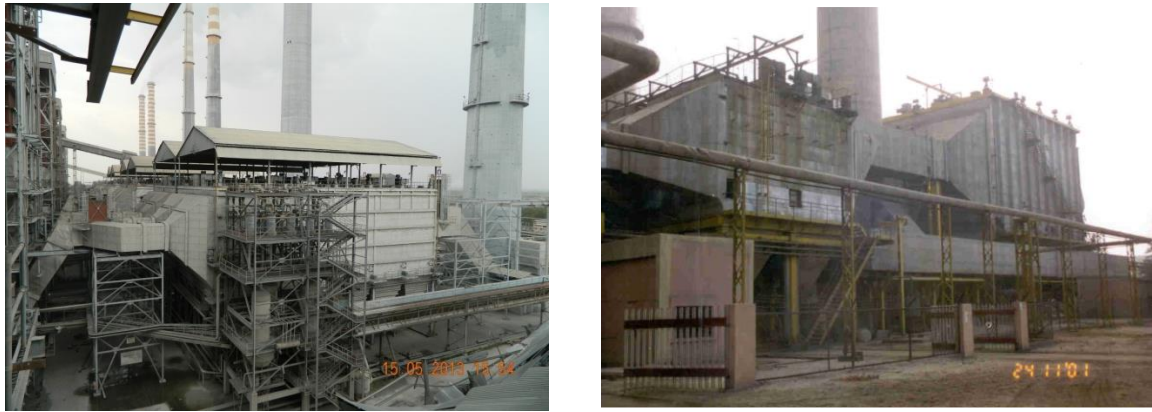
Fig.1: Electrostatic Precipitator at the Thermal Power Station
