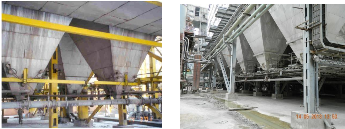
Fig.2: Structural steel supports of electrostatic precipitator
