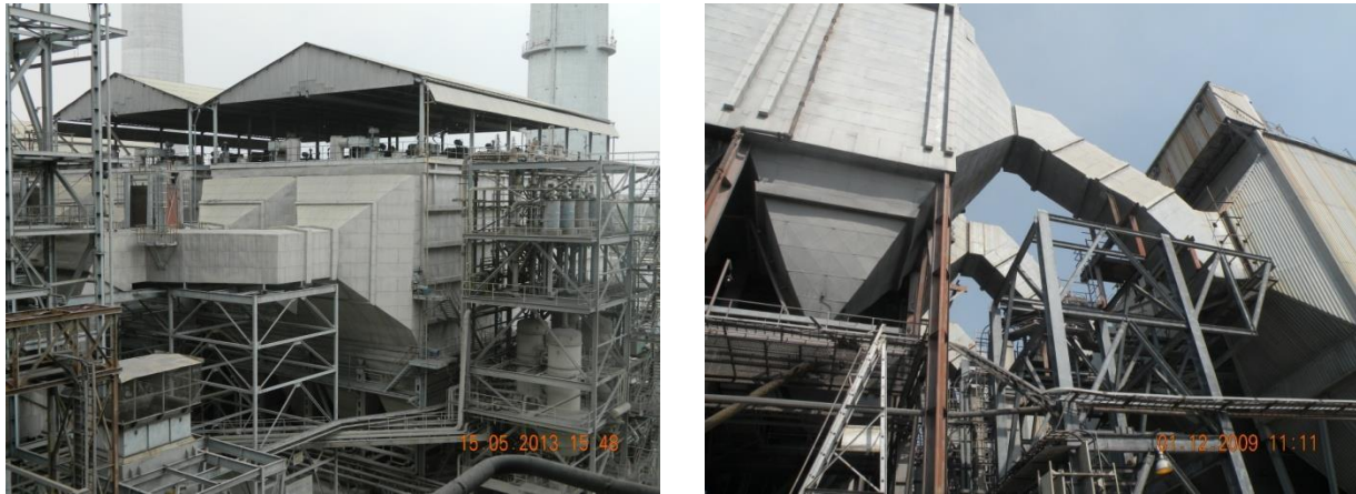
Fig. 3: Ductwork of the electrostatic precipitator
