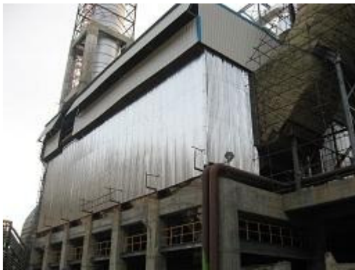
Fig. 9: De-dusting facility in India
