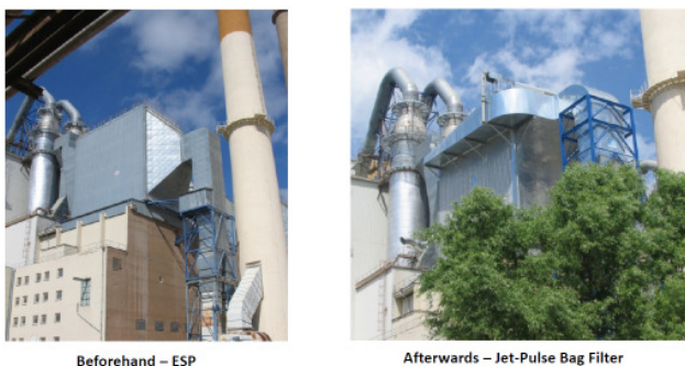
Fig. 10: Retrofit of an electrostatic precipitators to a Jet-Pulse bag filter
