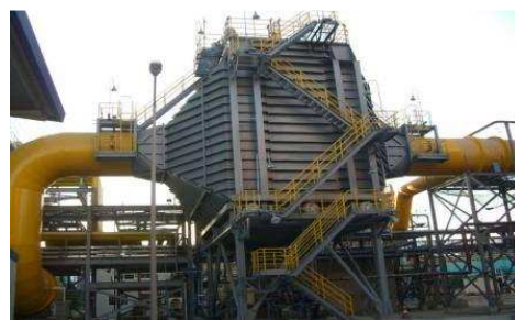
Figure 7 WESP for GTCC Plant in Korea
