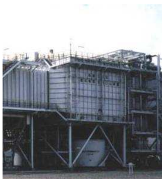
Figure 9 WESP for Coal-Fired Boiler in Japan
