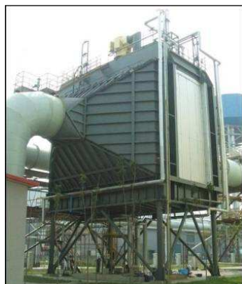
Figure 6 WESP for GTCC Plant in China
